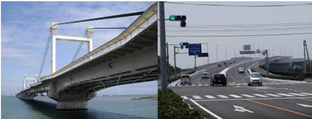
Fig-2 The Awa Shirasagi Bridge: Facility F(cable stayed bridge), Environment E(in traffic service)
